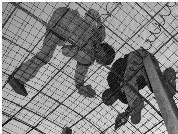
Tying off expanding metal lath on roof with pneumatic hog ring pliers.
